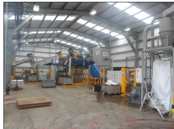
Fig. 2: RJ-ZZDB integrated into a PP Washing Line
